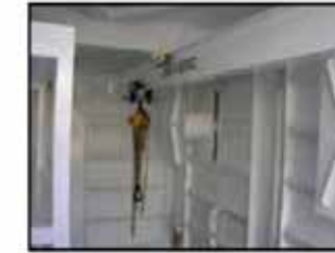
WORKSHOP WITH 1 TONNE HOIST / PULLEY SYSTEM
