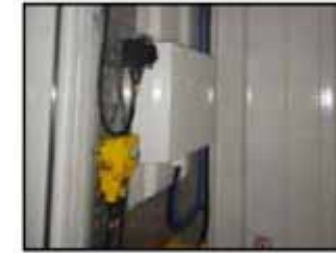
EXD SHUTDOWN SWITCH
